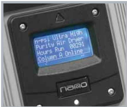
PLC controller with clear text display
